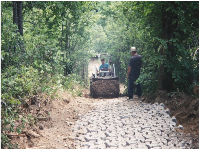
After the blocks are in place cover them completely with fill to a depth of about 2 inches.
