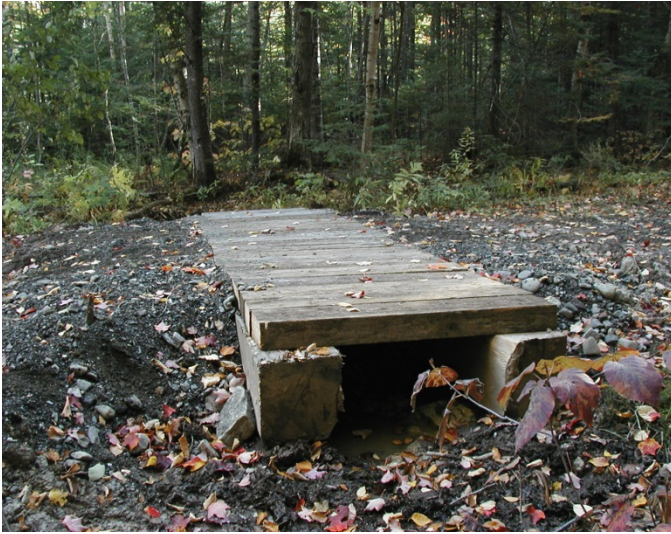
Box culvert: no gravel cover
