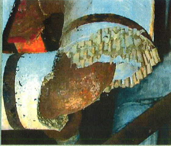
Damaged asbestos pipe insulation.
