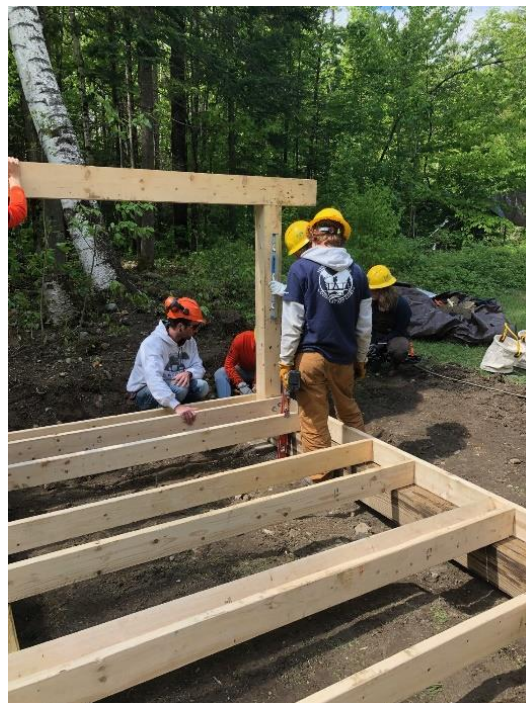
Carpentry Training at Moose Brook State Park. Members construct the frame for a camping shelter.
