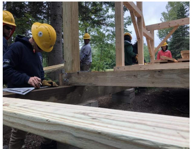
Carpentry Training at Umbagog State Park. Members construct the frame for a camping shelter.
